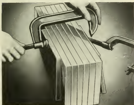
1. Sand boards smooth and glue together. Use casein-base, cold glue, sold at most hardware stores. Make block 6 \times 6\frac{3}{4} \times 17 in.
